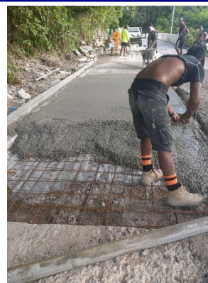
The infrastructure department repair damaged road and will resume painting road markings
